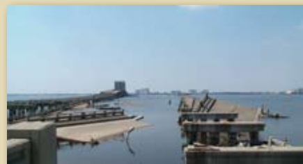
Hurricane Katrina damage to bridge
